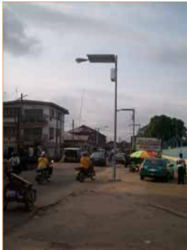
Sol's new TSL Series installed along roadway in Nigeria, Africa
