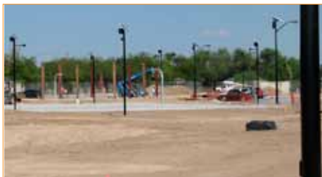
Greenway™ and TPM systems installed at South Tower Park in Alamo, Texas
